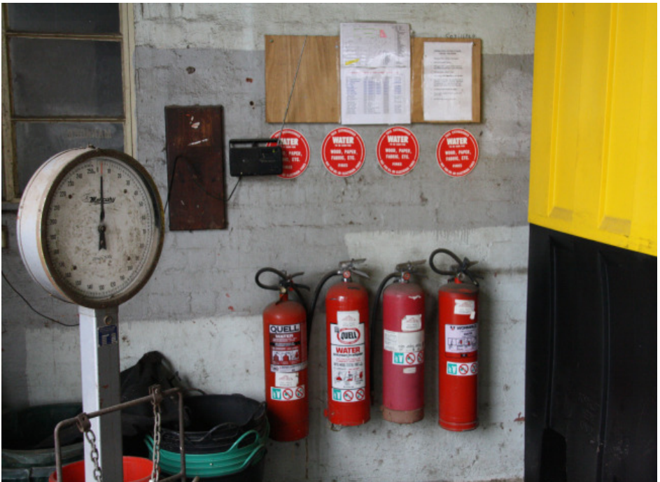
Bottom: Fire Preparation in a feed room
